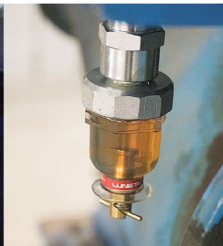
Large Blower - Wastewater Treatment Plant
