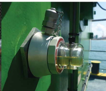
Mooring Winch - Ocean Dredger
