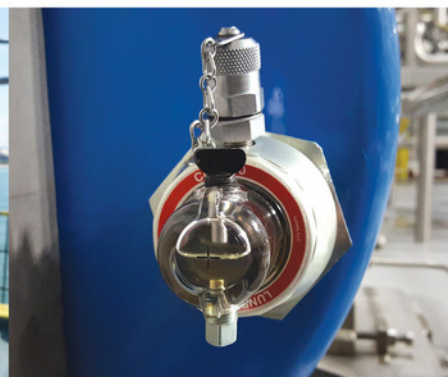
Screw Pump - Bottling Plant
