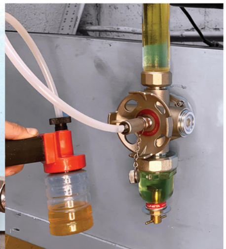
Pulling an Oil Sample
